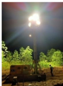
Gambar 2. Towerlamp 12 meter terpasang lampu LED NL500D.
