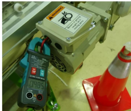
Figure 4. Direct measuring of the load current
